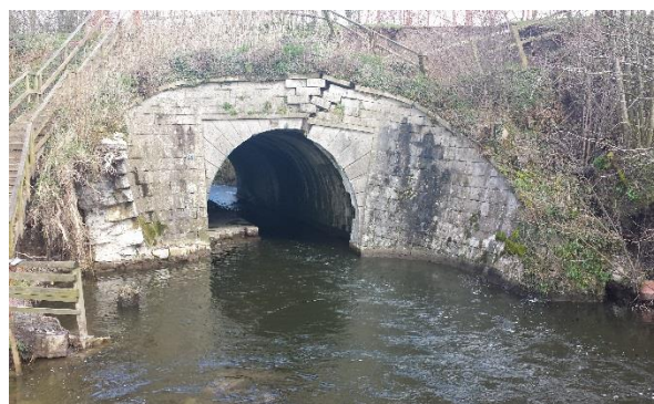
Severe damage caused by Storm Desmond December 2015
