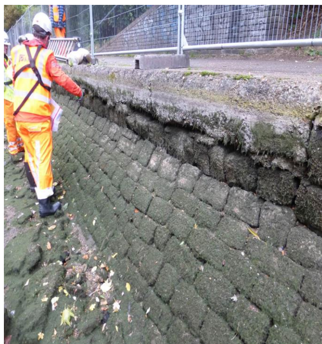
Regents canal waterway wall repairs featured in publicity for start of winter works programme
