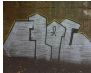
Graffiti – an ever present problem on waterway structures
