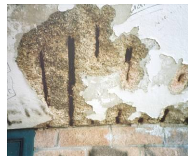
Carbonation of concrete leading to spalling and exposure of corroding reinforcement
