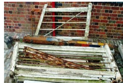
Defective paintwork leads to wet rot in timber
