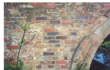
A patchwork of poorly matched bricks, mortars and 'plastic repairs'
