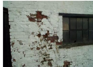
19 th century brickwork painted with inappropriate modern masonry paint
