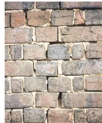
Loose mortar, open joints – a wall in need of repointing
