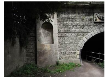
After removal by chemical cleaning
