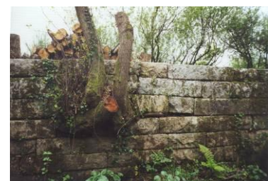
Disruption caused by vegetation
