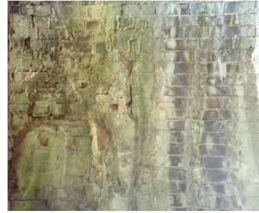
Lime wash out and salt efflorescence on the underside of an arch
