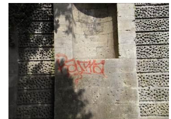
Graffiti on Bath stone, Grade II* listed asset
