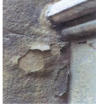
Calcium sulphate blister caused by pollution
