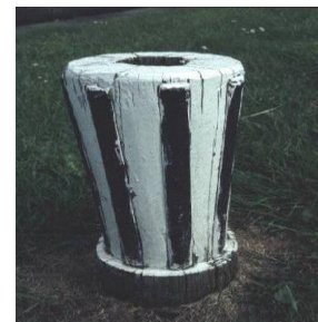
Paint looks shipshape, but it can lead to rotting timber
