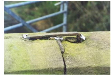
Damage caused by iron cramp
