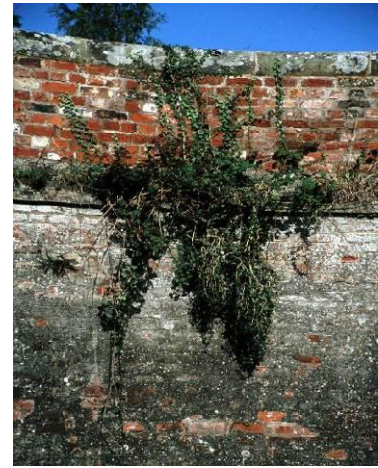
Organic growth can cause problems
