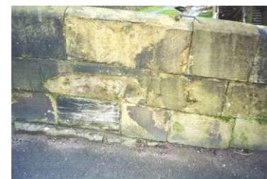
Stones fixed in wrong bedding plane
