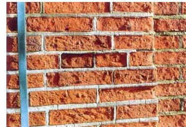
Spalled brickwork due to use of hard cement mortar
