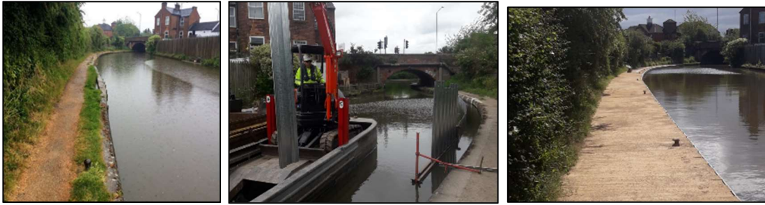
Before, during and after photographs of the piling and towpath works through Leamington on the Grand Union Canal
