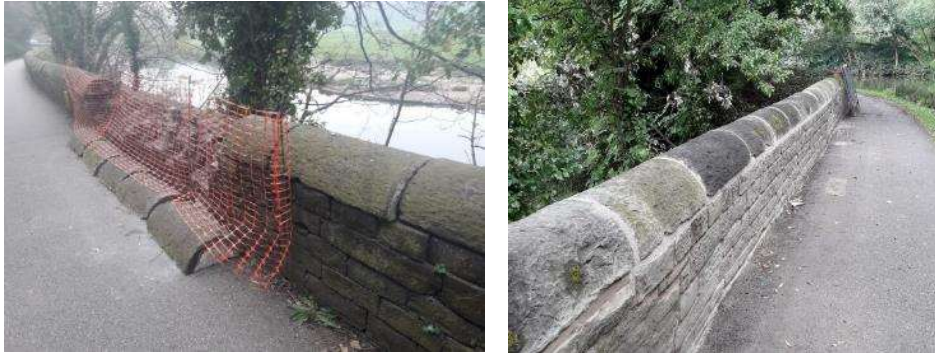
Boundary wall bulging on Embankment 5, Brookfoot To Ganny on the Calder & Hebble Canal
