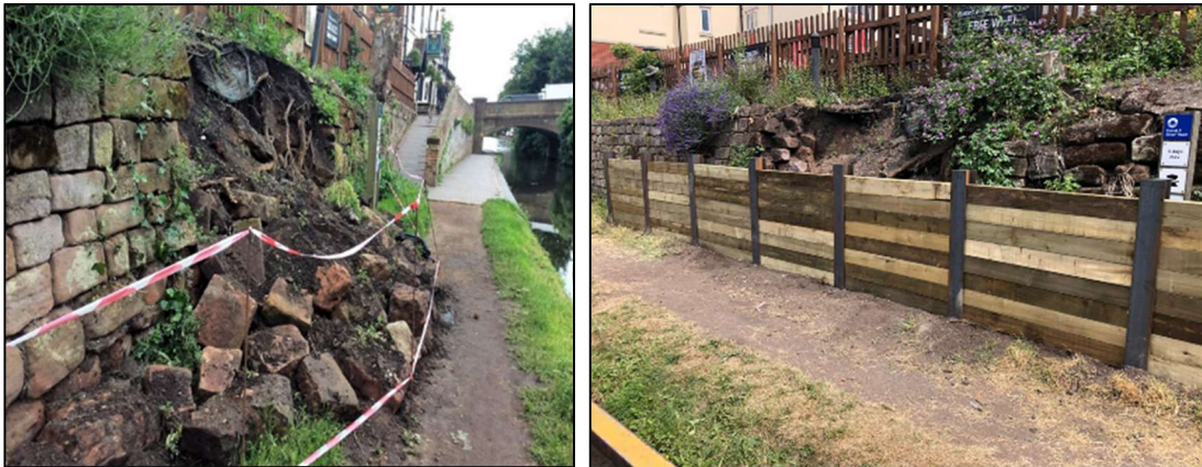
Emergency works to collapsed retaining wall in Stourport on the Staffs & Worcester Canal. Work completed by Direct Services and the West Midlands Region Reactive Team.
