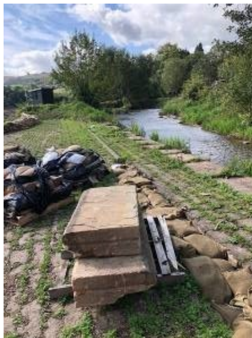
Main spillway weir and bywash channel (weir blocks removed during the incident)
