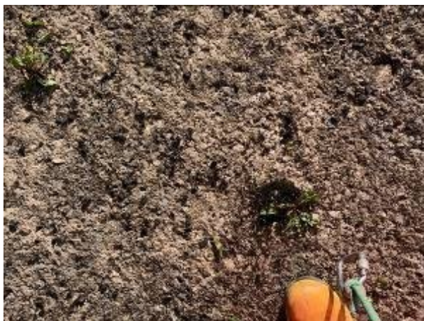
Blocked relief wells
