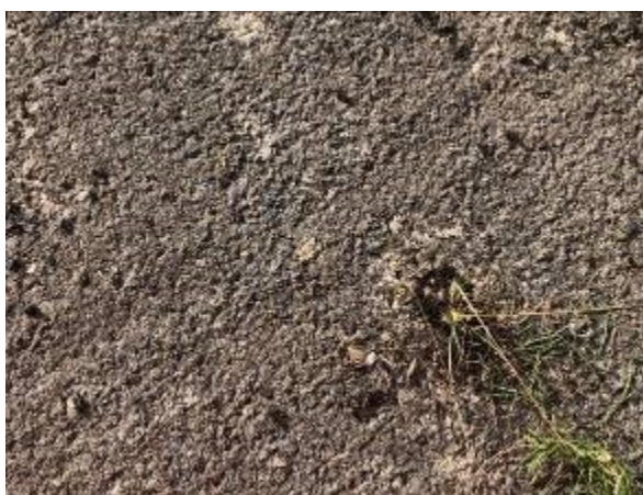
Blocked relief wells
