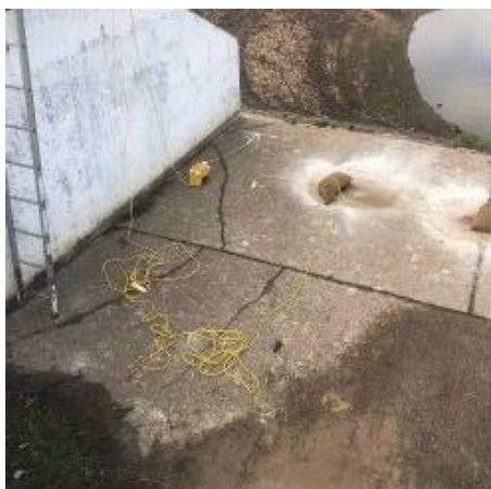
Cracking at extreme left end
