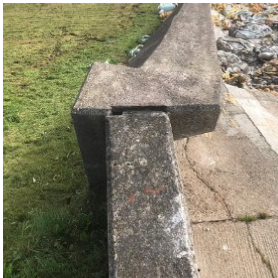
Crack to spillway
