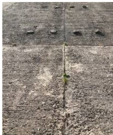
Blocked relief wells
