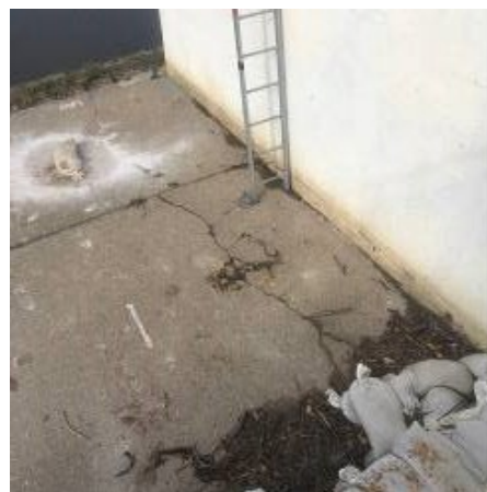
Increased cracking at left end
