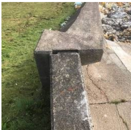
Movement between spillway and wall
