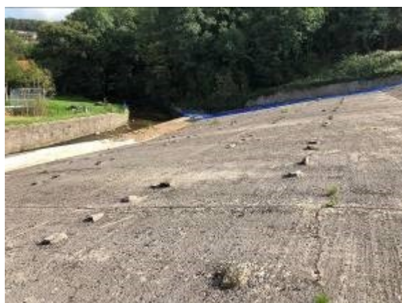
Crack to spillway
