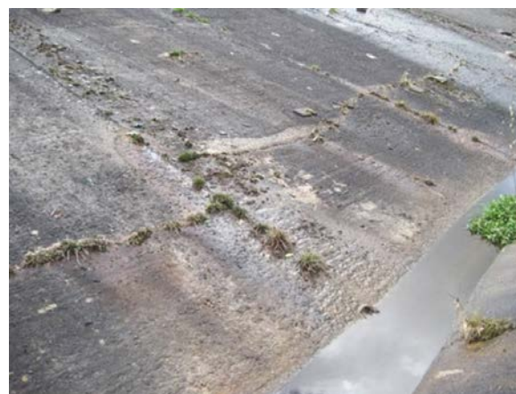
Accumulated water at the base of the spillway
