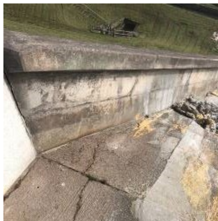
Movement between spillway and wall and cracking
