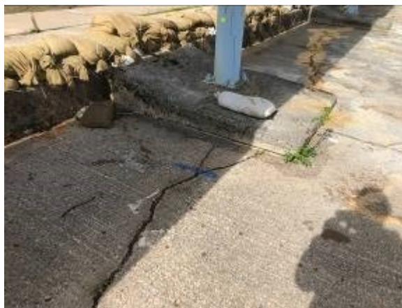
Cracking to crest
