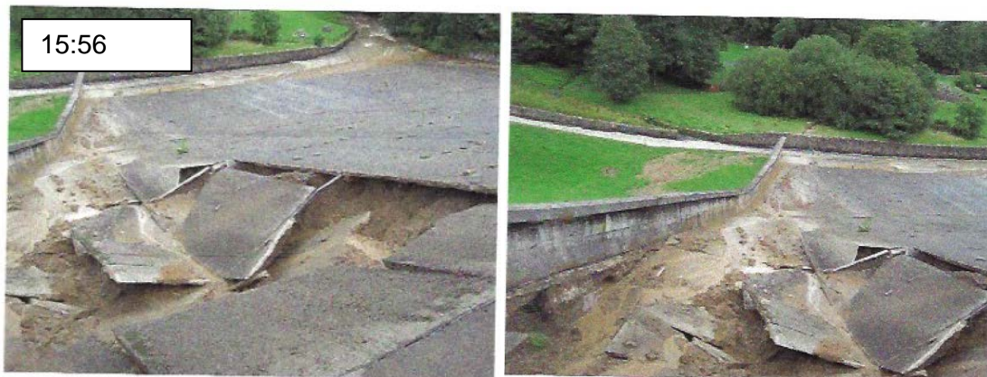
Slabs collapsed into enlarged void
