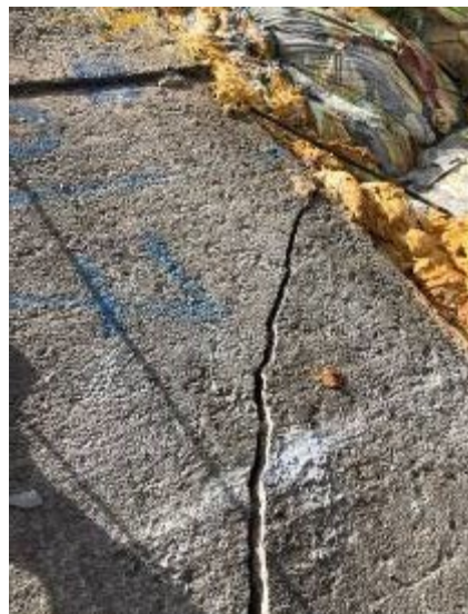
Crack to spillway
