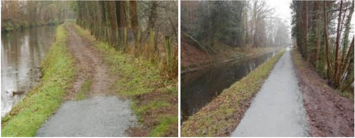
Upgrade of 7km of towpath at 3 sites on the Mon & Brecon Canal
