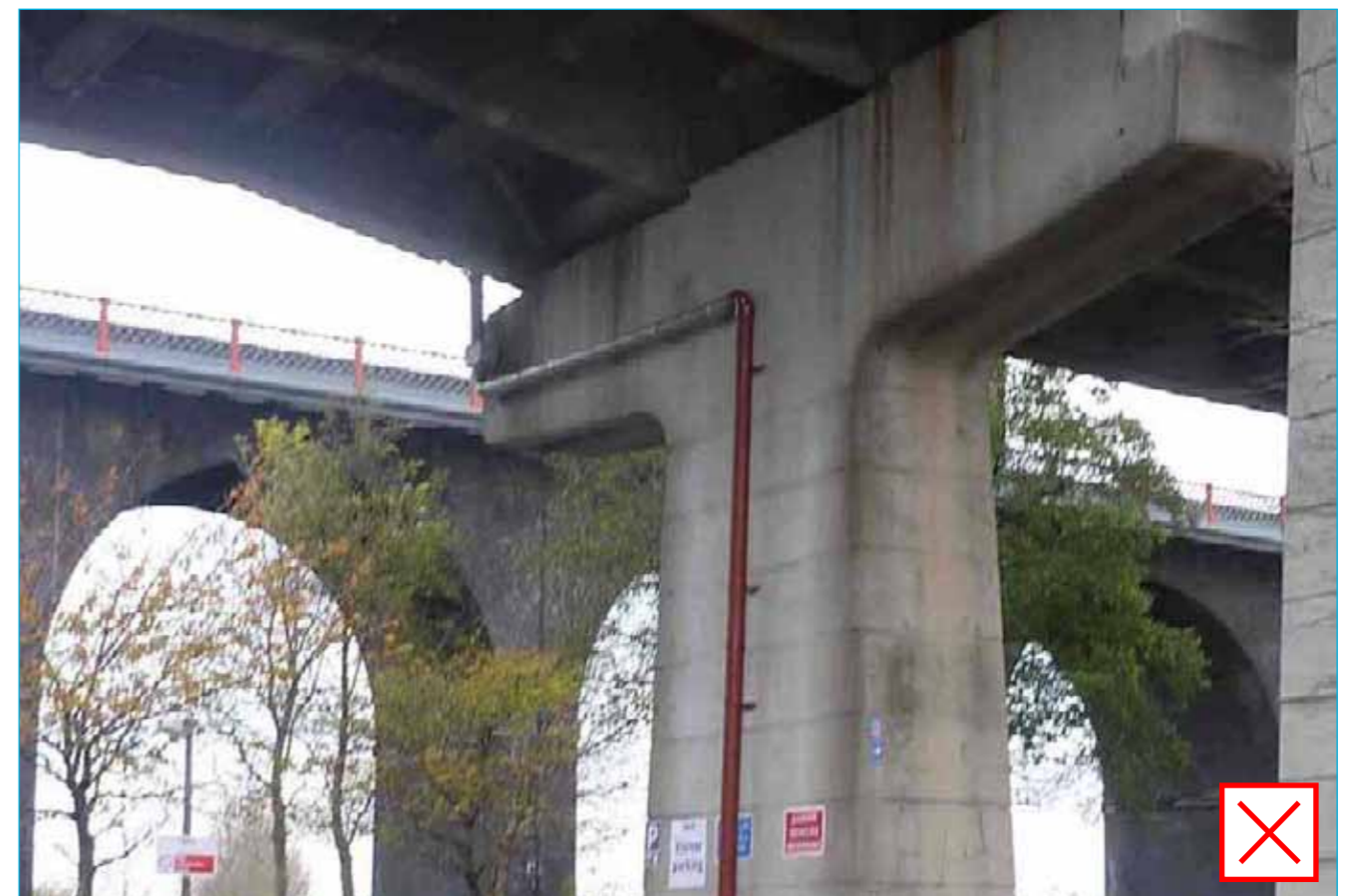
Fig.B16.4 - Poorly designed drainage appears ill-considered and unsightly
