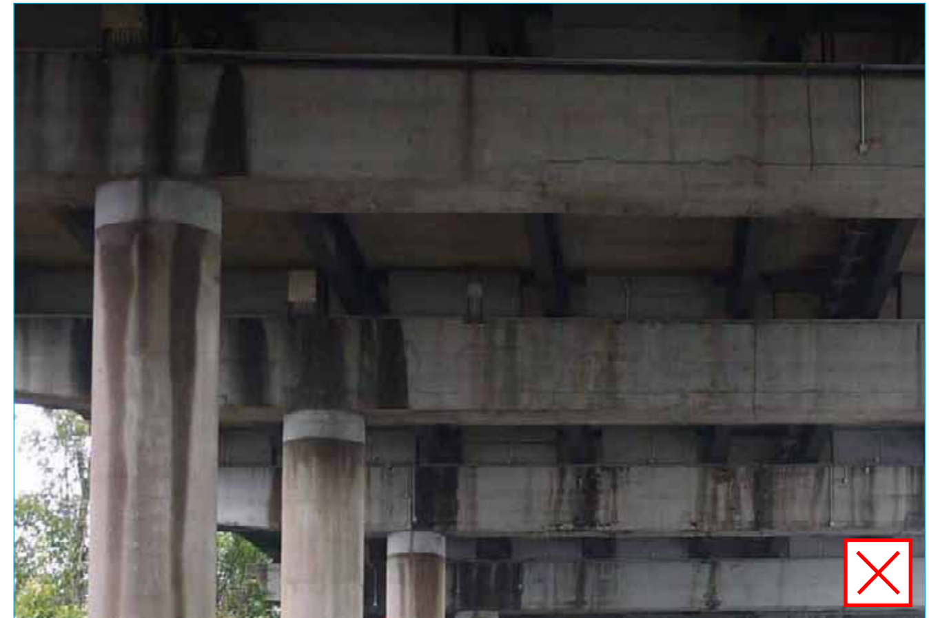
Fig.B15.1 - Poor quality, stained concrete is unacceptable
