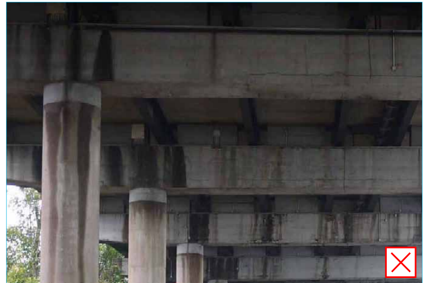
Fig.B15.1 - Poor quality, stained concrete is unacceptable
