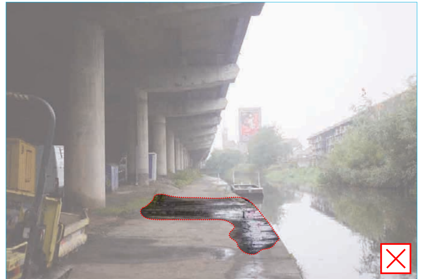
Fig.B16.3 - Poor drainage details impact on the towpath beneath
