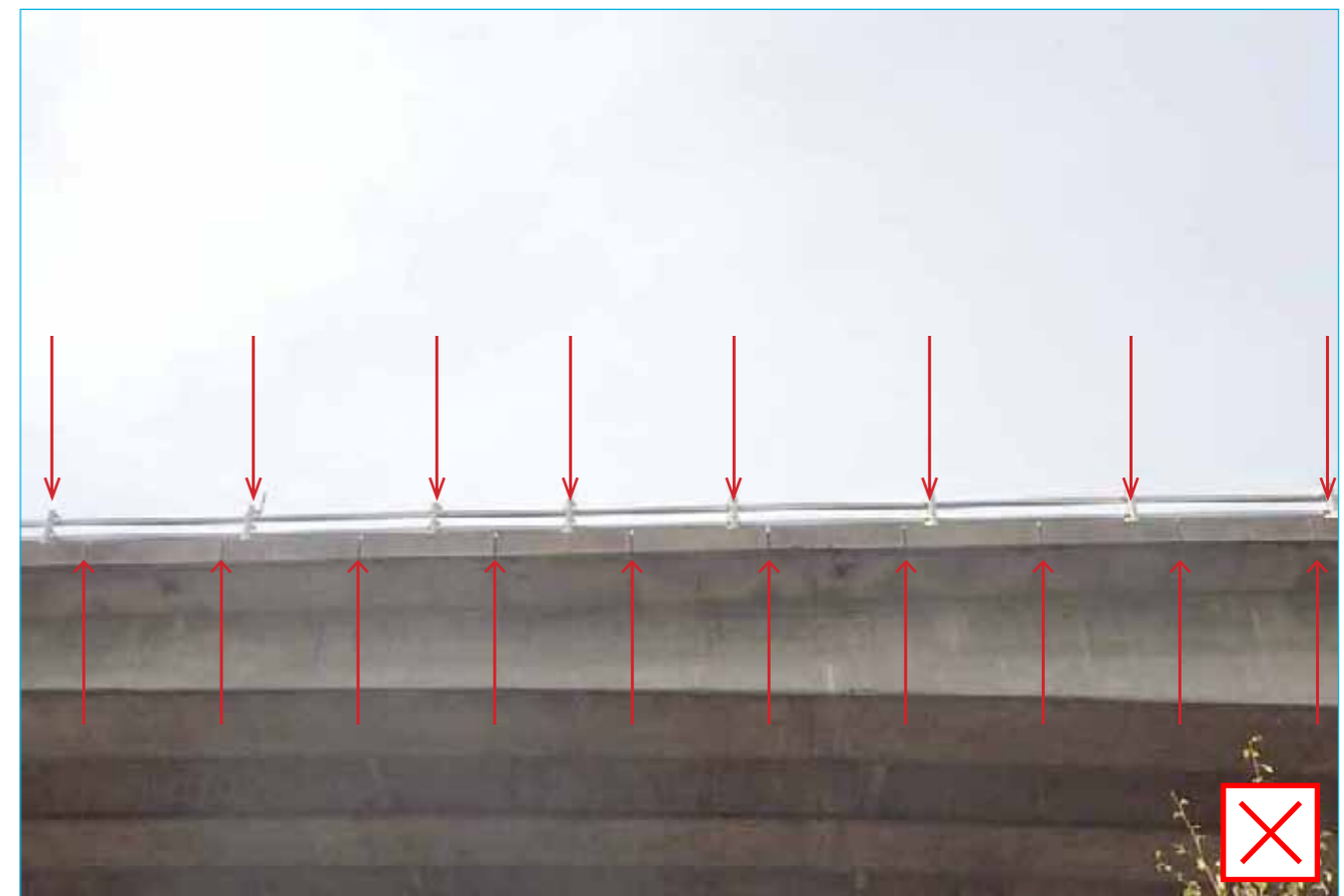
Fig.B16.2 - Poorly coordinated elements appear ill-considered and unsightly
