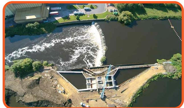
Hydropower plant at Knottingley
