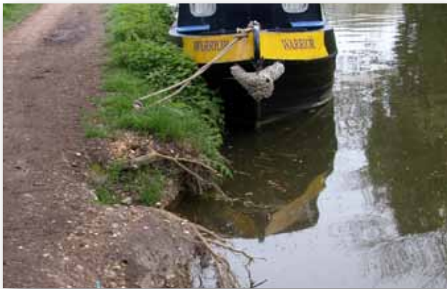
The edge of the canal can be washed away by the flow of water
