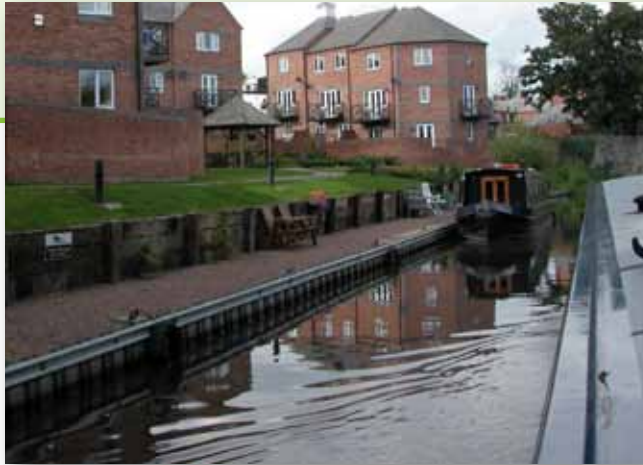
This stretch of waterway in Kidderminster has been lined with steel piles to make the banks strong
