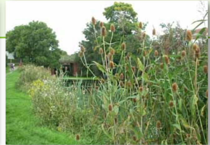
Waterside plants growing at the canal edge act as a buffer and stop moving water from wearing the bank away
