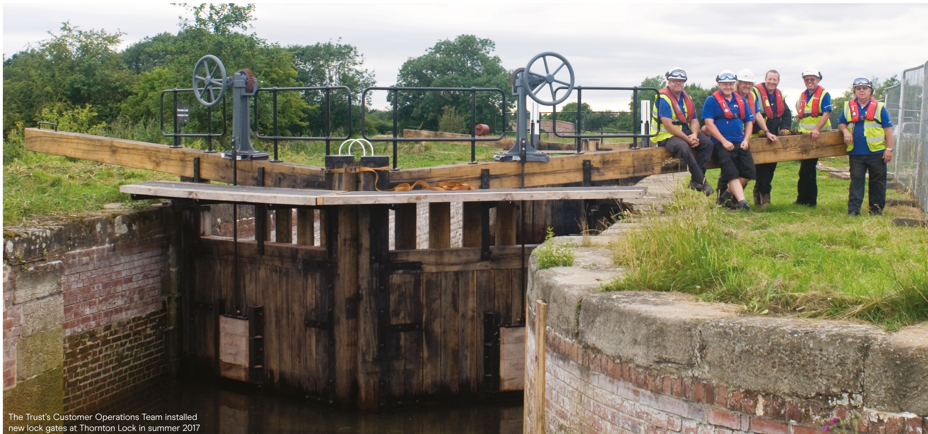
Trust contractors Land & Water dredging below Top-Lock in November 2017, made possible through Heritage Lottery Fund support.
