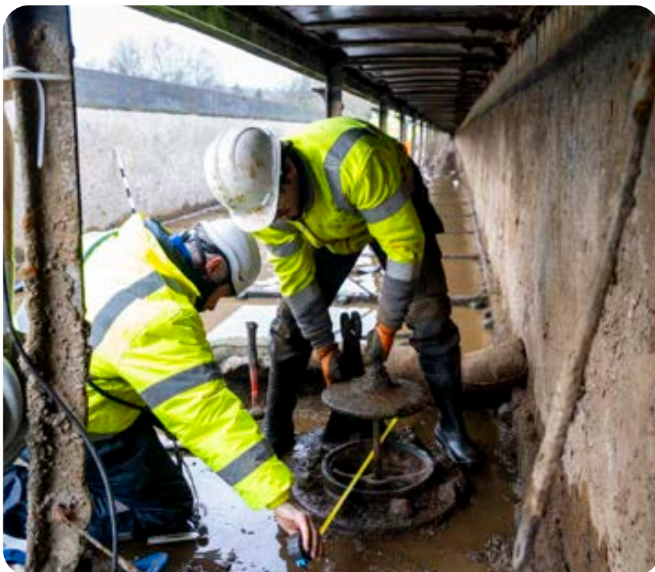
Left: In 2024 we drained the Pontcysyllte Aqueduct, enabling our engineers to carry out a full inspection for the first time in 20 years. And our year-long 'The Bridge that Connects' cultural programme celebrated communities within the Pontcysyllte Aqueduct World Heritage Site by sharing stories of the area. The project was funded by Shared Prosperity Funding through Wrexham County Borough Council.
