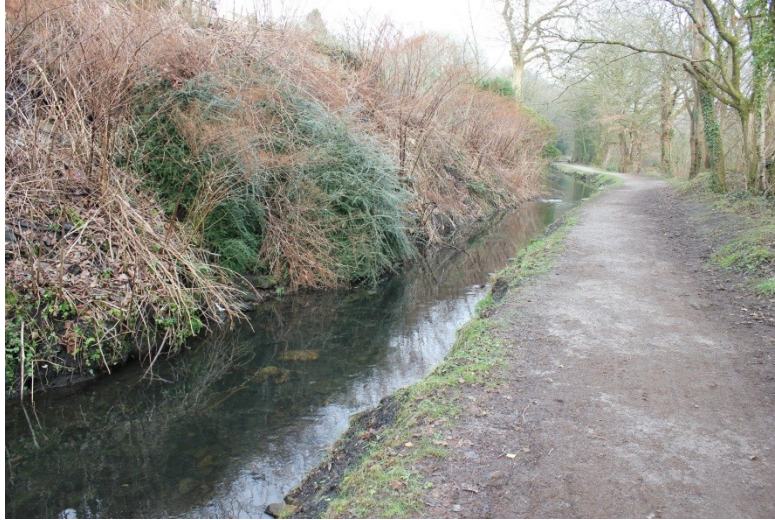
Image 9: Encroachment near Trebanos
