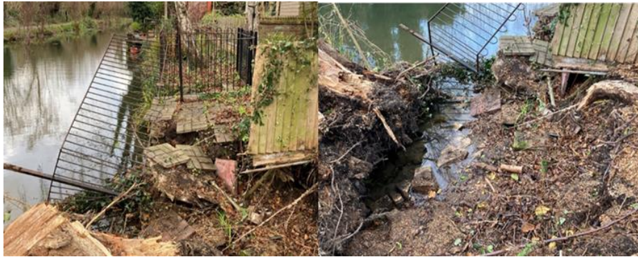
Photo: Oxford Canal, slip and damage caused to offside gardens
