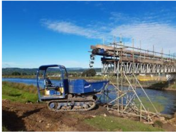
Conveyor system at Altham Embankment (Leeds & Liverpool Canal) which kept Canal live for boaters, avoiding a weight limited bridge on a fast dangerous country road, plus the need for traffic management and daily road sweeping.
