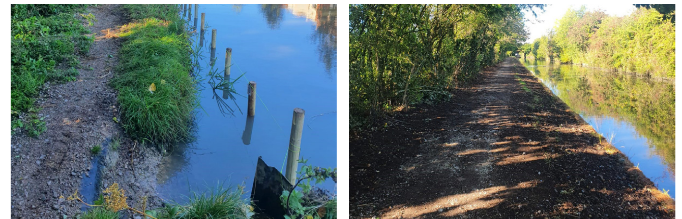
Photos of the canal bank before and after the bank stabilisation works
