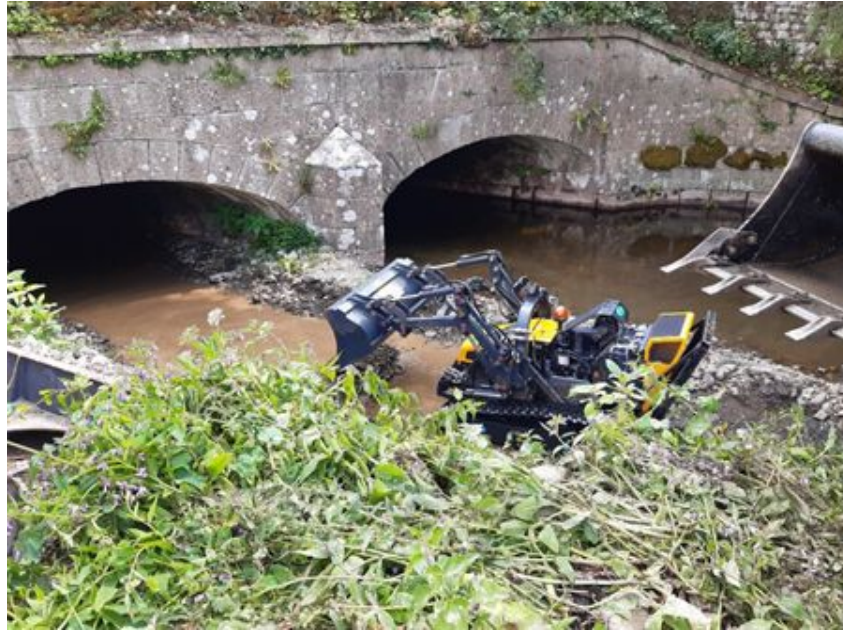
Peasey Beck clearance works on the Lancaster Canal using remote controlled loader
