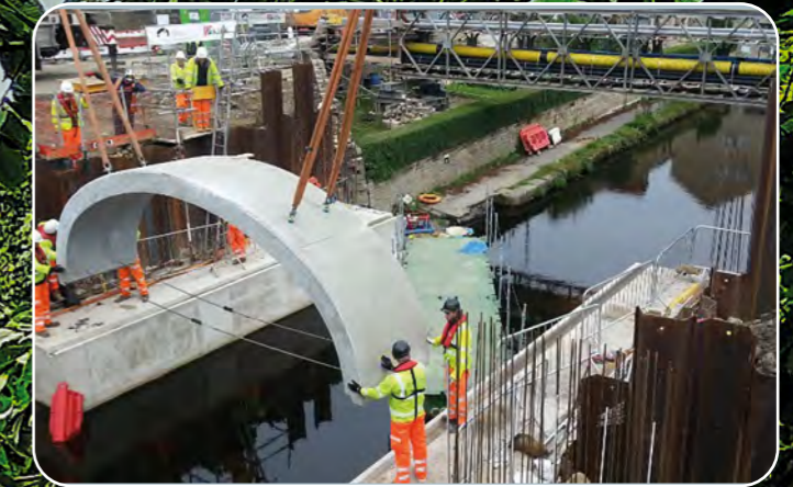
The Boxing Day floods of 2015 were so severe that Smeaton's Elland Bridge could not be saved and had to be carefully demolished.
