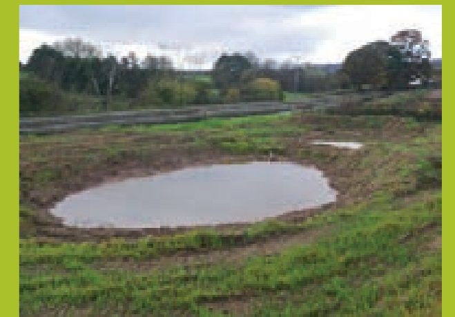
Ponds being constructed on the Montgomery Canal to create new great crested newt breeding habitat, once the vegetation is well established
