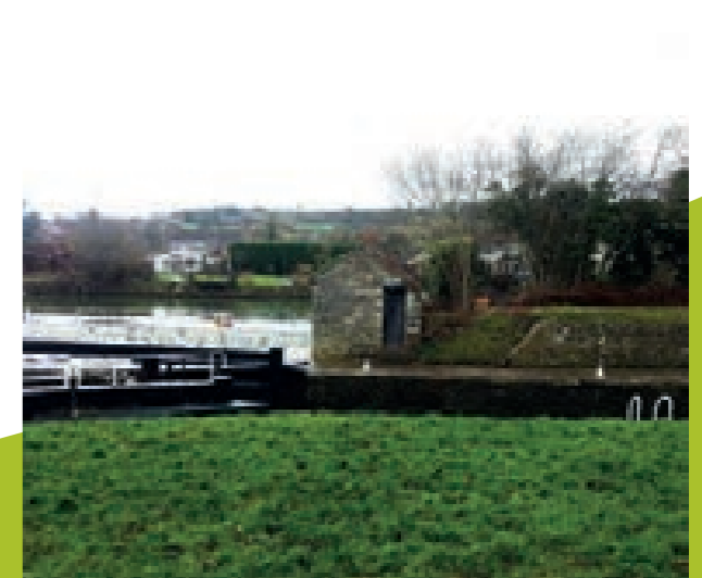
Bat grille on lock hut allowing bats through but stopping disturbance from people
