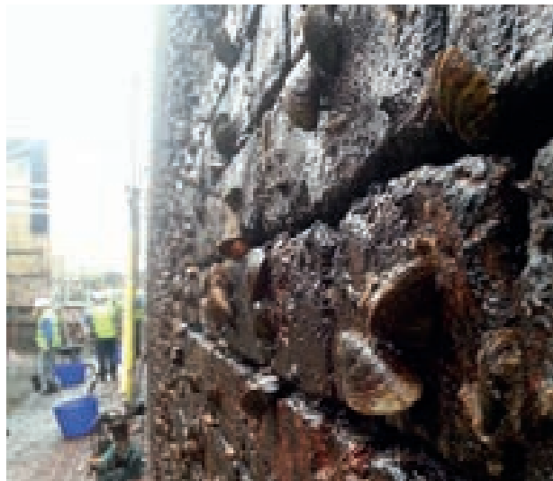
Zebra mussels on wall of drained lock during lock gate replacement work
