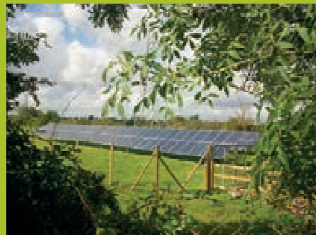
Solar panels help power the pumps to move water to the top of the Caen Hill Flight
