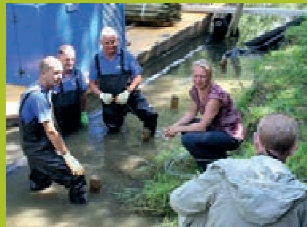
Ecologist working with Canal & River Trust construction team to install below water level Nicospan
