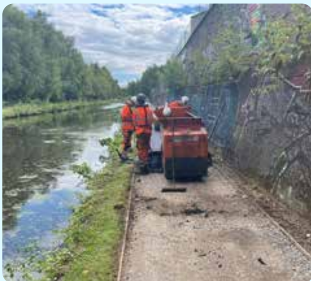
Towpath improvement works in progress (2023) between Birmingham and Sandwell, illustrating the delivery challenges these schemes can face.
