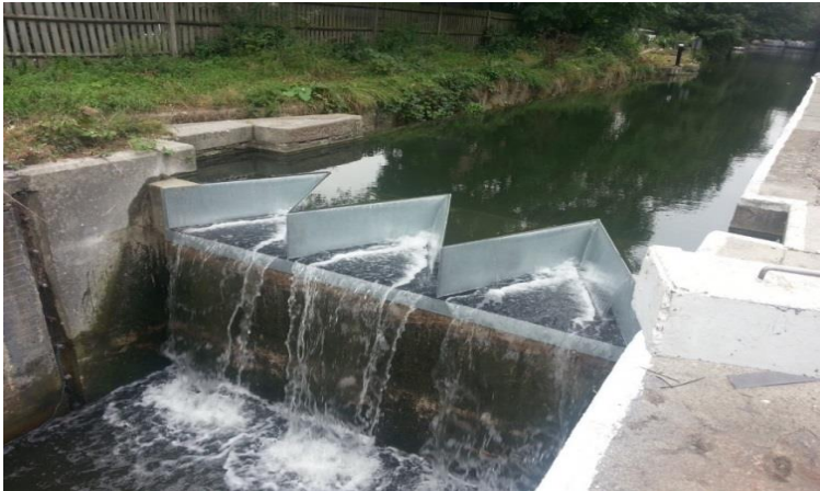
Surface Water Discharge
